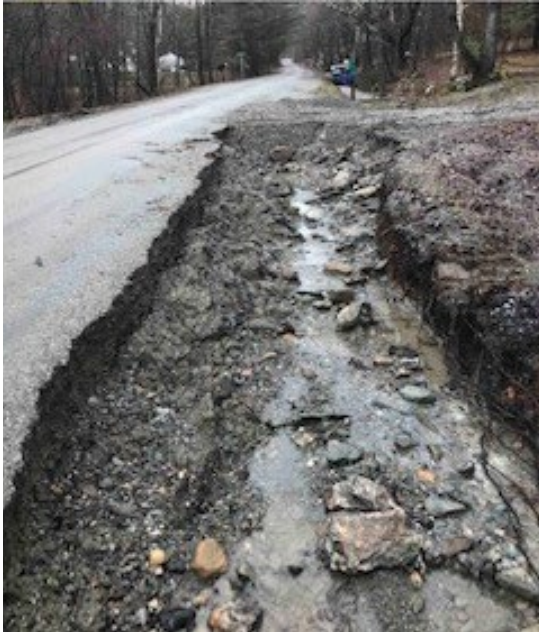
Road flood damage on Belgo Road during April 2019
