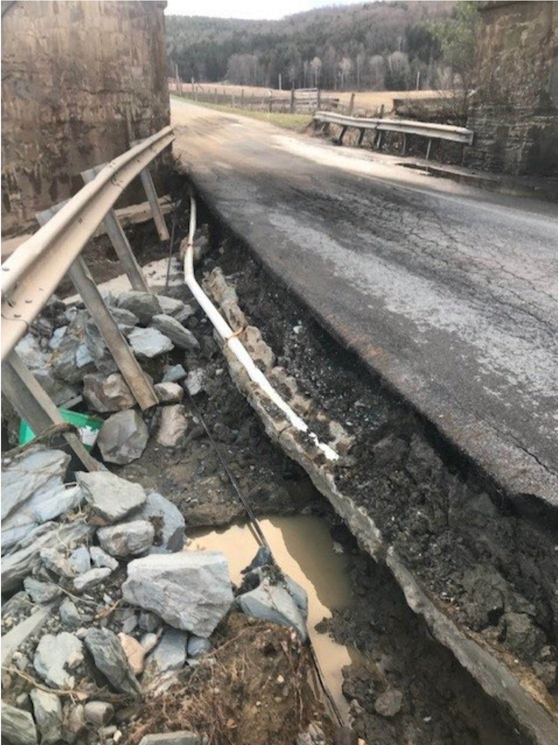
South Street Trestle Bridge Washout – April 2019
