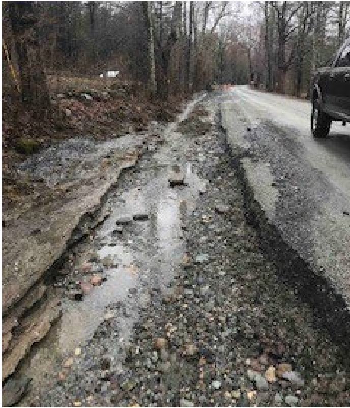
Belgo Road Flash Flood Damage – April 2019
